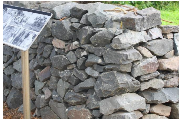
Figure 21 Basalt/ bluestone is a key characteristic of Kiama and has been integrated throughout the public domain
